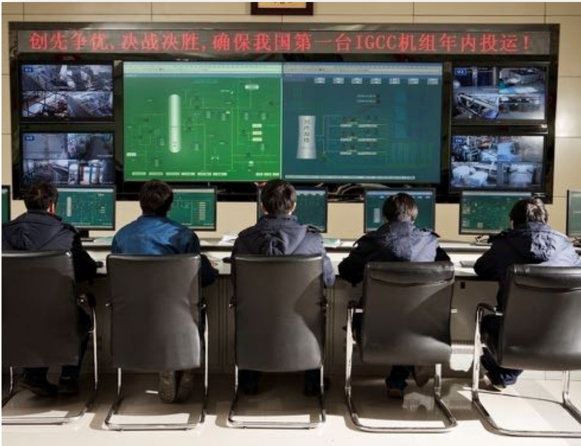
Control Room at the GreenGen Plant Tianjin, China
